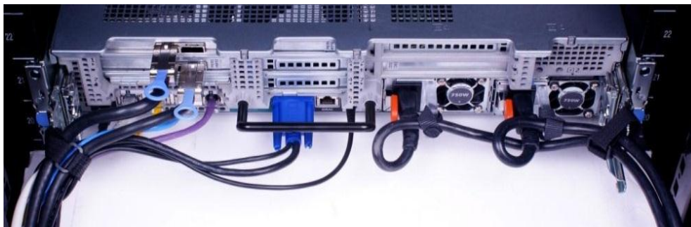
Figure 9. Cable routing without a CMA
